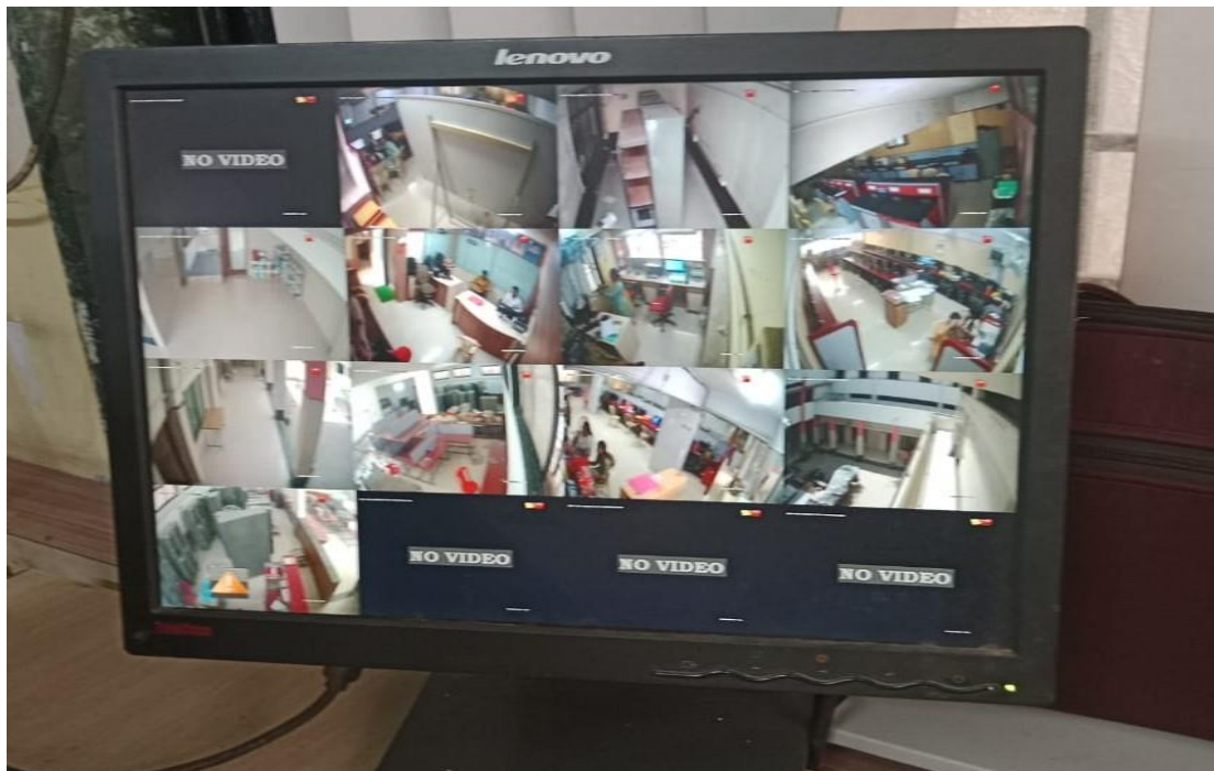
Continuous CCTV surveillance of the premises.
